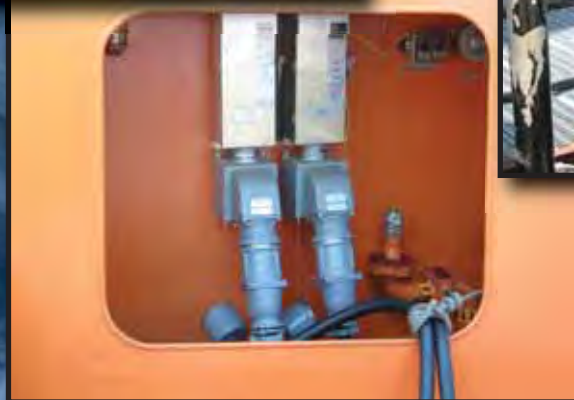
200A MaxGard inlets with disconnects
