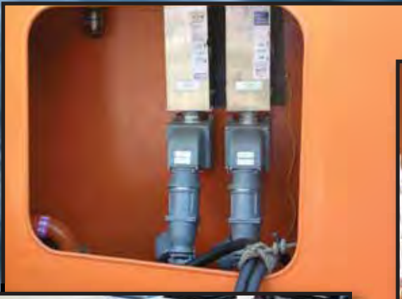
200A MaxGard inlets with disconnects
